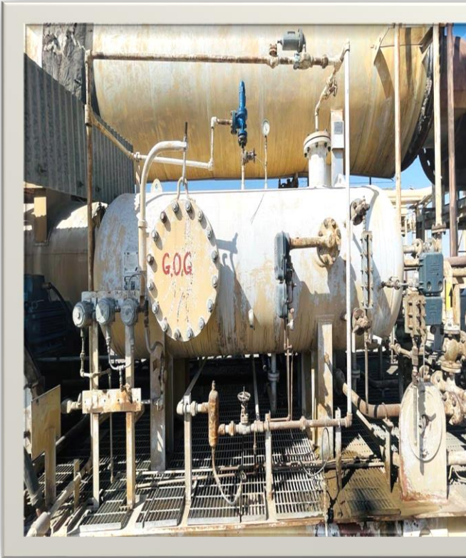
Figure 14: Glycol oil Separator(G.O.G)
