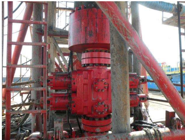
Figure: (4-4) PRESSURE CONTROL EQUIPMENT
