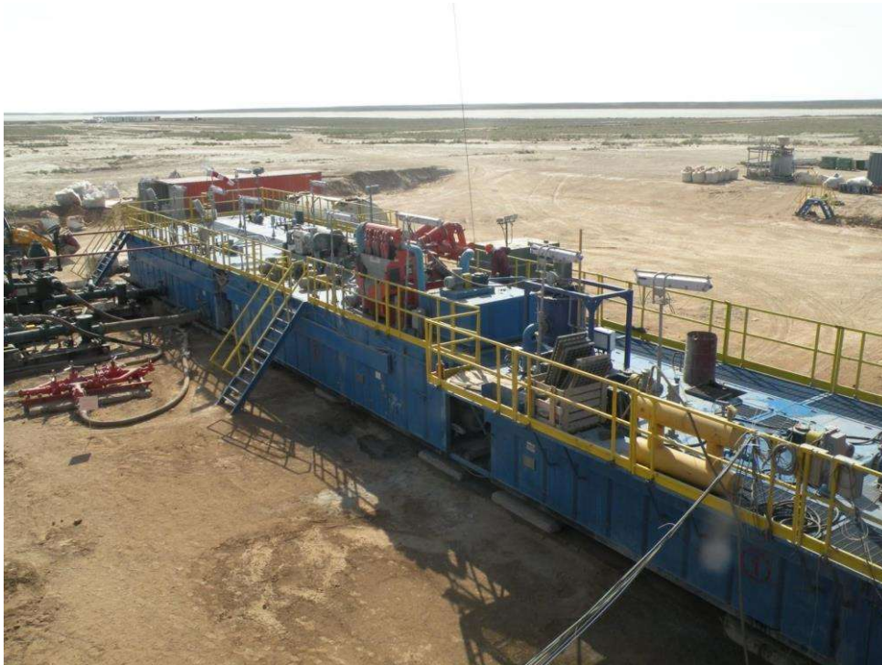
Figure: (3-7) MUD PITS AND SOLIDS CONTROL EQUIPMENT
