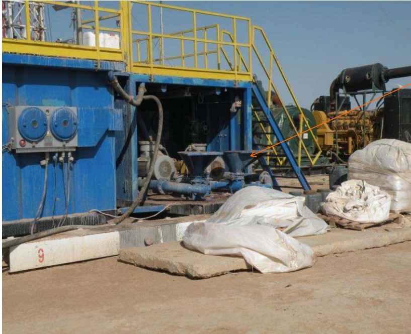
Figure: (3-8) MUD MIXING HOPPER
