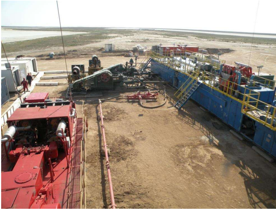
Figure: (3-5) MUD PUMPS
